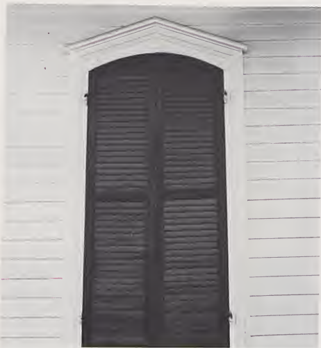
A window frame of the Fisher Gatekeeper's House. The Wainman, Winn and Fisher homes used identical exterior millwork, perhaps obtained from the W. C. Petty Company in Archdale.
