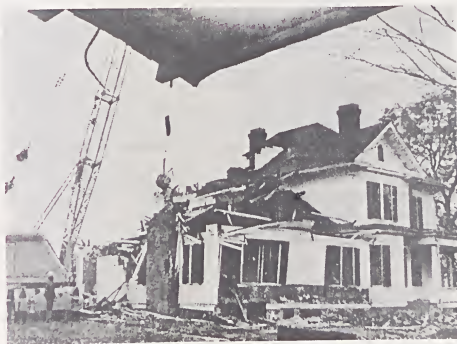
One of the last survivors of Asheboro's Fayetteville Street residential neighborhood is destroyed in 1973. Attempts to convert the W. J. Armfield house into a county museum were unsuccessful and the site was developed for commercial uses. Originally known as "Elliott's Green," the park-like corner lot was the site of the Asheborough Female Academy in 1839.
