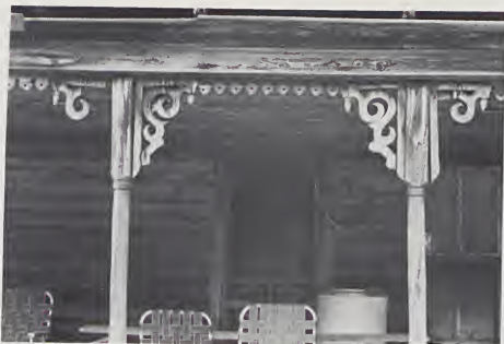
Detail of house in Coleridge Township showing sawnwork brackets, turned porch posts and pierced sawwork soffit decoration.
