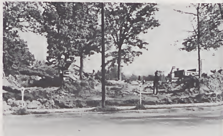
(G) Gone. The hilly lot is being leveled; the Randolph Savings and Loan building, Asheboro's first modern multi-story building, would soon rise on the site.
