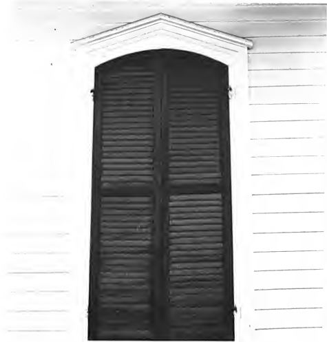
A window frame of the Fisher Gatekeeper's House. The Wainman, Winn and Fisher homes used identical exterior millwork, perhaps obtained from the W. C. Petty Company in Archdale.
