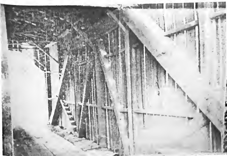
Documentary photograph showing the interior construction of the Skeen's Mill covered bridge, an example of mortise and tenon construction.
